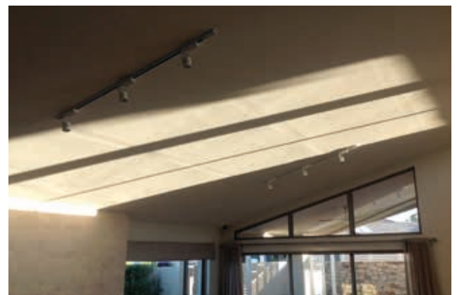
Figure 6: Same plasterboard surface under glancing light
